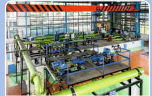
Advanced Pump Testing Setup and Calibration Lab
